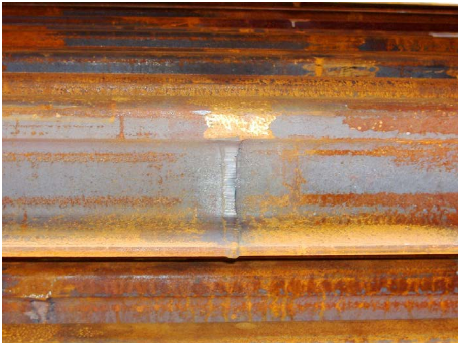
Stationary Flash-Butt Weld on Long Rolled Bhilai, SAIL, Rail; pict. by F.A. Wingler
