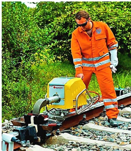
Modern Digital controlled AT "SmartWeld" High Quality Rail-Welding by Th. Goldschmidt`s Digital controlled Process
