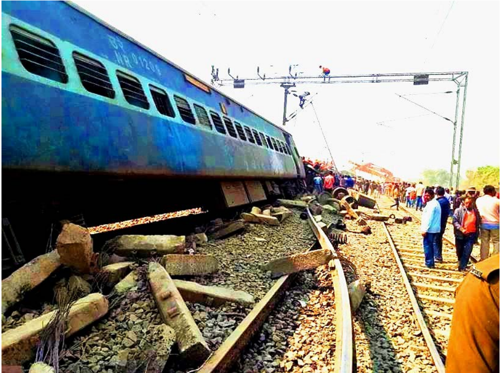
Fatal Seemanchal Express Derailment due to a Rail Fracture in Vaishali District, Bihar, 03-02-2019
