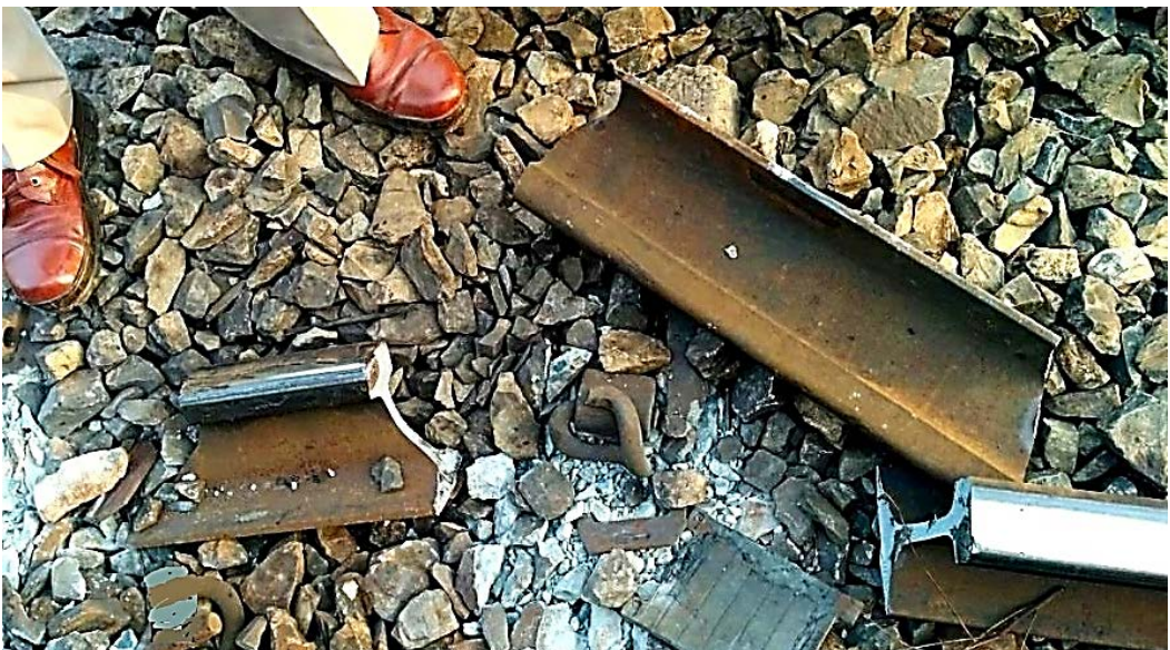
Rail-Weld and Rail-Head Defects leading to fatal and nasty Derailment Disasters on IR
