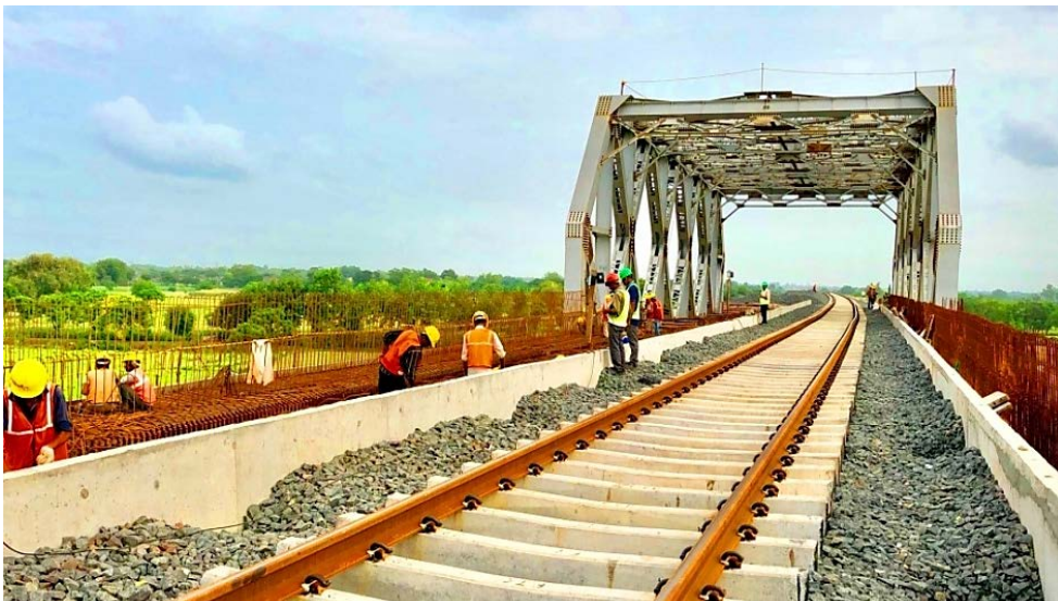
Ongoing Construction Works on India's Eastern Dedicated Freight Corridor with LRR-CWR Track; photo: Joe Qian/World Bank
