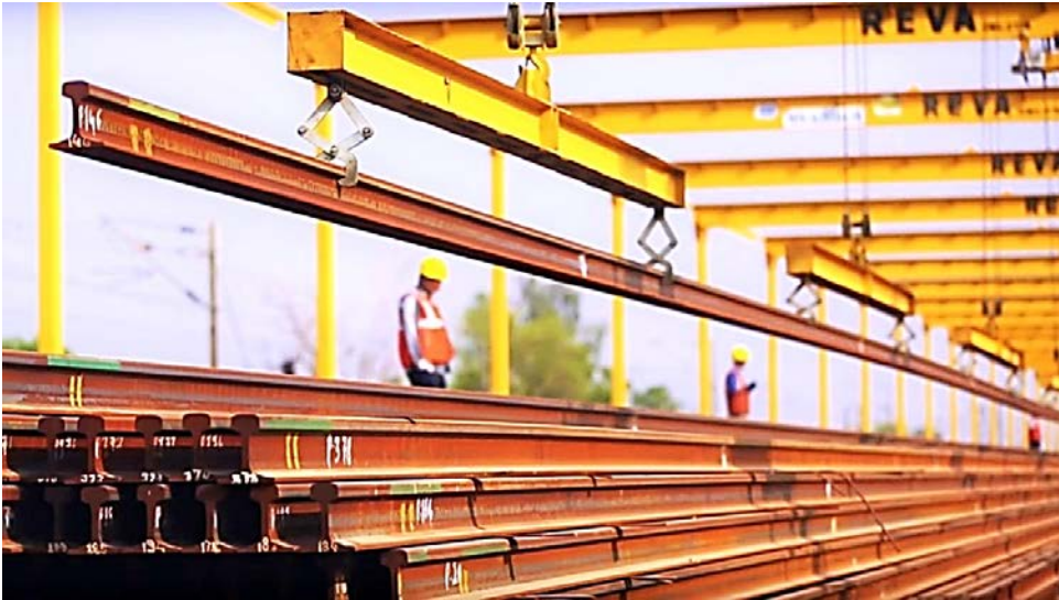
Picking-up of Long Rolled 60 kg Rails, LRR, for Dedicated Freight Corridor, DFC, with synchronised Cranes; India
