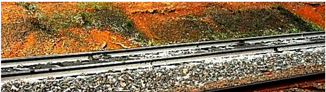
Fig. 11a: White Marks on “dancing”/badly packed Concrete Sleepers caused by Ballast Abrasion
