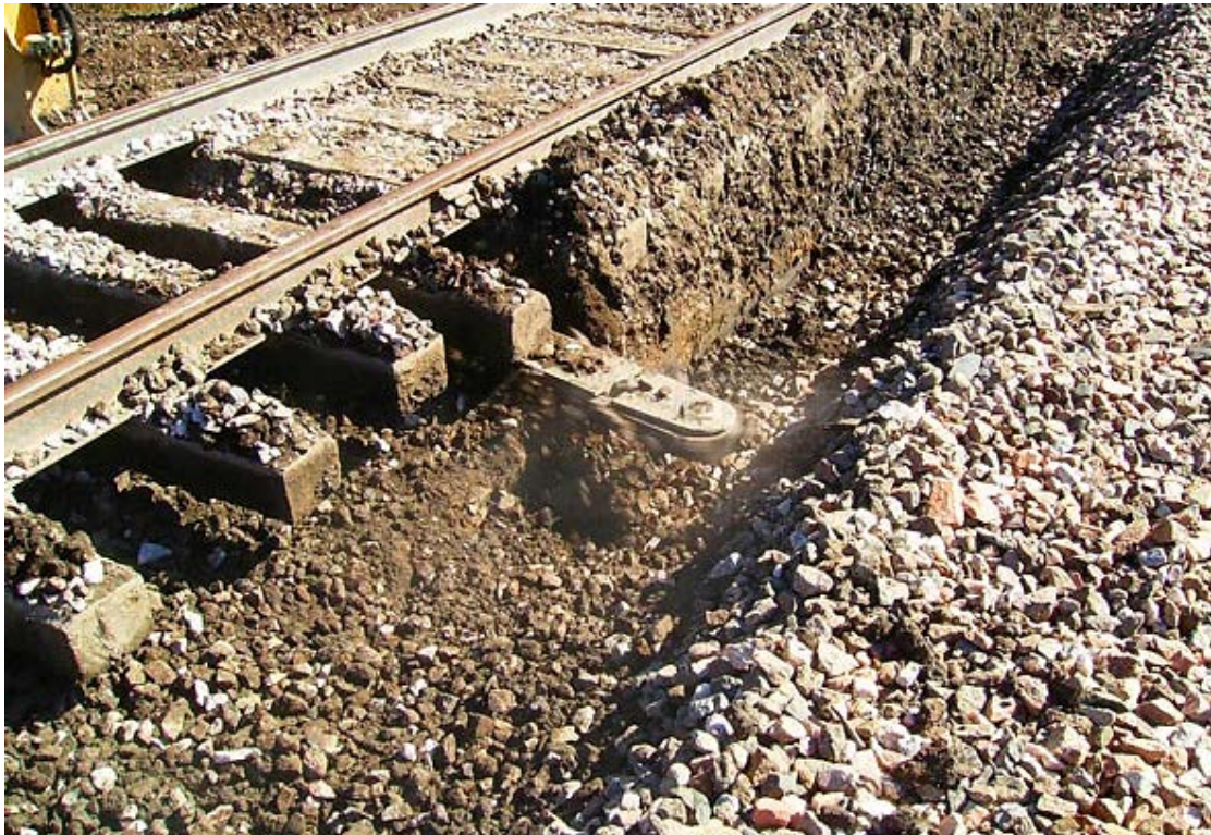
Fig. 15: Removing Mud and Muck from under the Sleepers with Off-Track Under-Cutter; Pict. by Hulder
