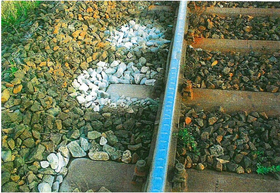
Fig. 11b: White Ballast Stones created by “dancing” Sleepers in poor packed Ballast-Bed: Pict. by IBES Baugrundinstitut GmbH
