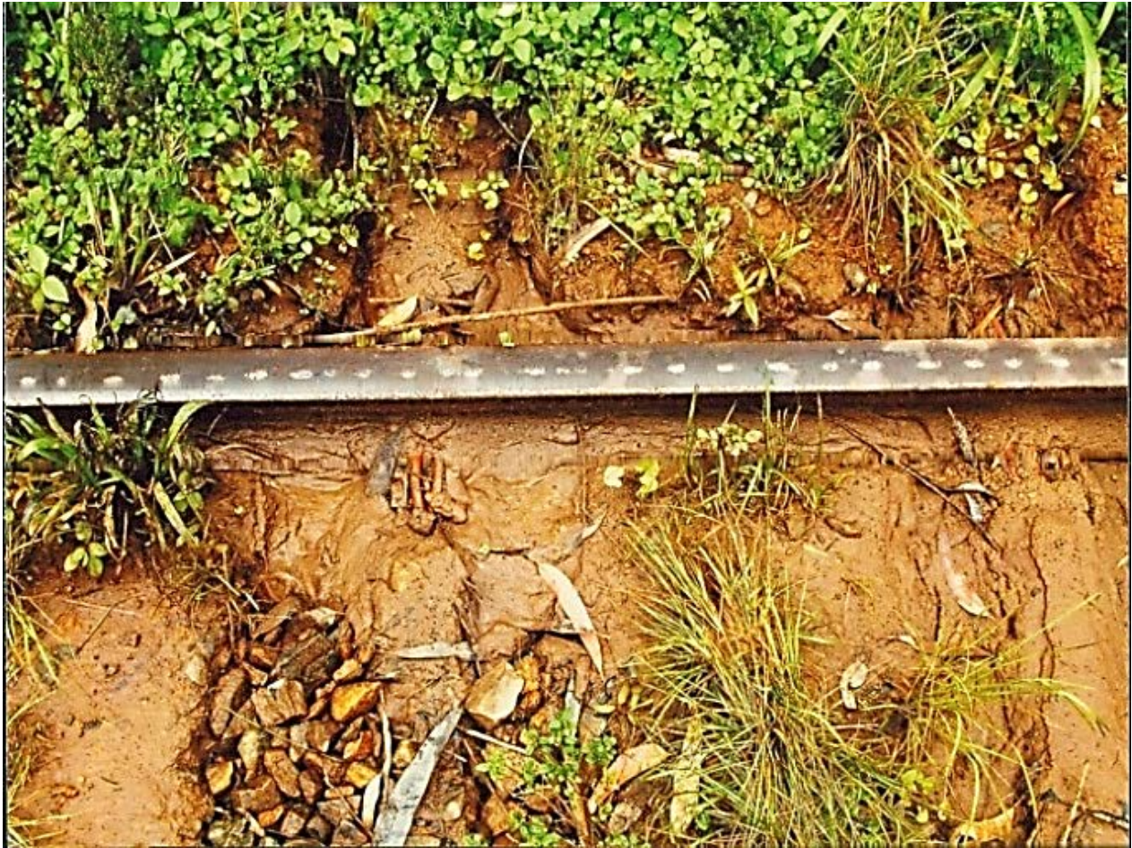
Fig. 6: Result of Laying new Steel-Sleepers without clean Ballast on UWA Line, Rozella-Hatton; the “dancing and tilting” Steel-Sleeper crush the Formation Material into Mud and submerge; Pict. by F. Wingle
