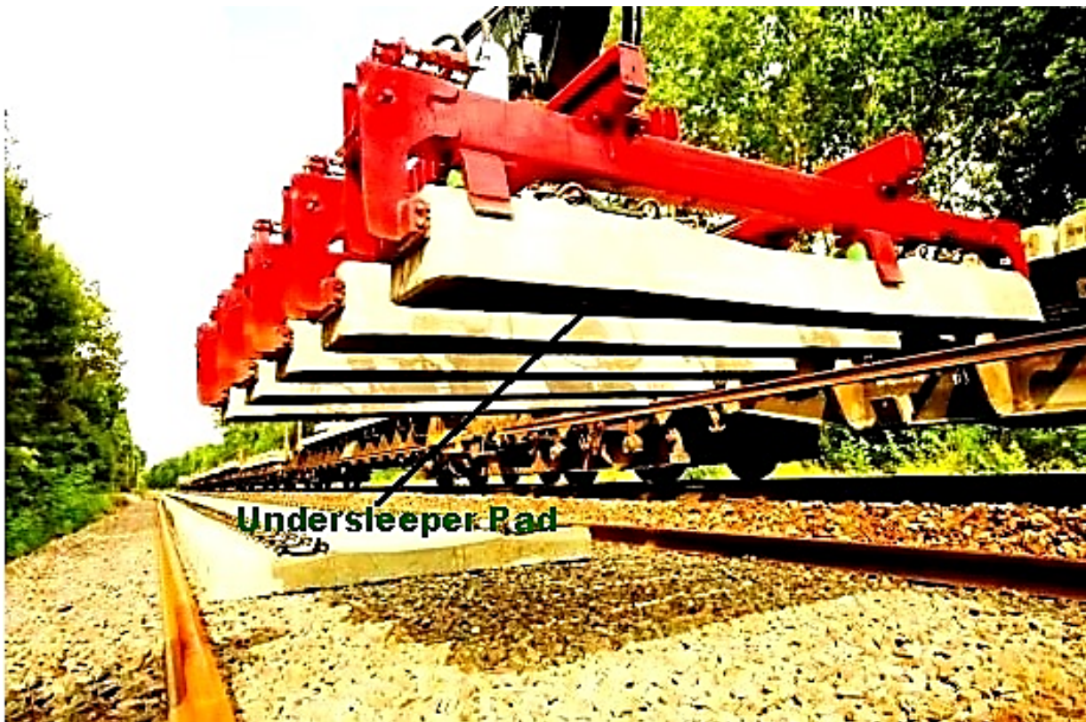
Fig. 4a: New laid Concrete Sleepers with Under-Sleeper Pads; Pict. by Getzner, Austria
