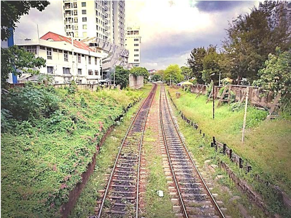
Fig. 1: Typical poor Quality Srilankan Rail-Track with nearly no Ballast on poor bearing Formation; Pict. from Ceylon Railway Forum
