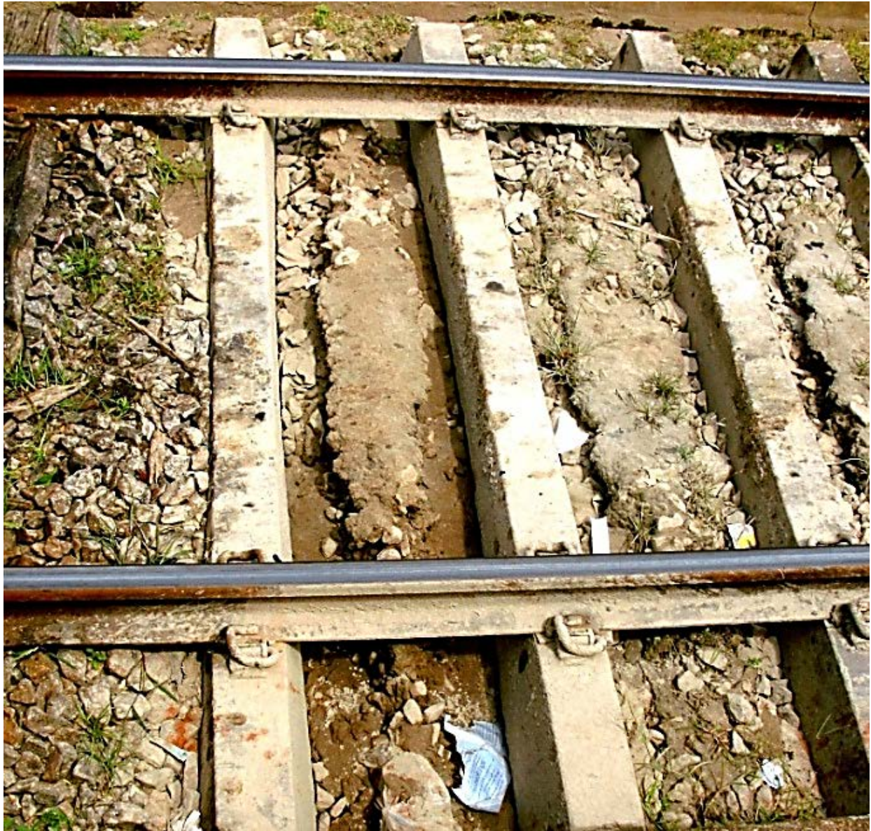
Fig. 10: Result of insufficient Ballast Depth and fouled Ballast causing Formation Damage on SLR Track; Slurry rises up through the Ballast and Ballast-Stones submerge into the Formation; Pict. by F. Wingle
