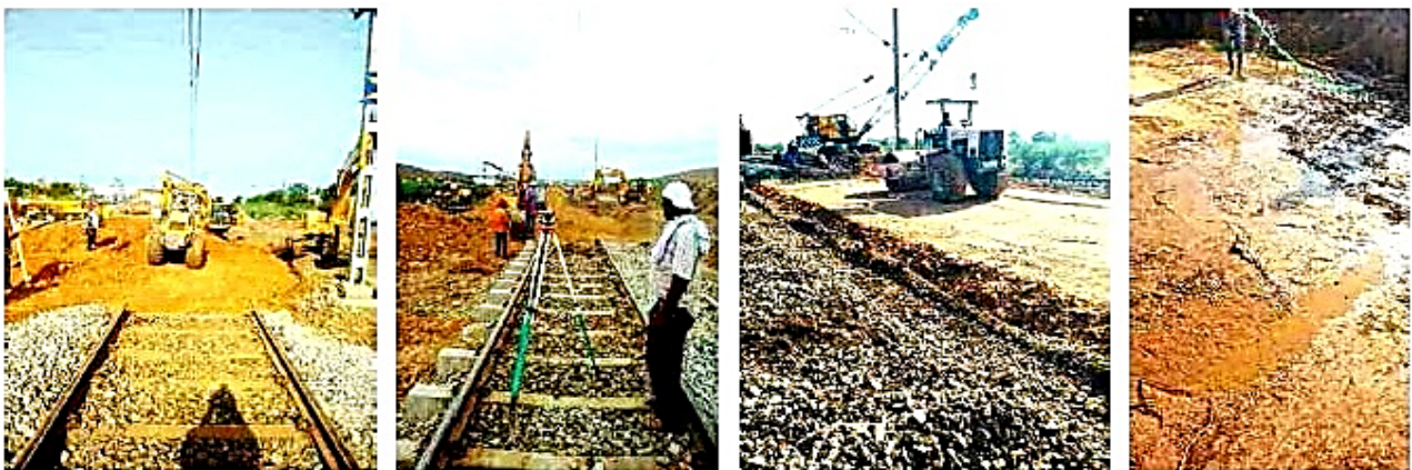
Fig. 19: Formation Rehabilitation with conventional Off-Track Machinery under Traffic Block with complete Track-Removal; see paper No. 23 on Formation Treatment with Moorum.... , presented by T. Anil Kumar, S. Veerama and U. Sarath on IPWE International Seminar, 23-24 th Febr. 2018, at Guwahati, India
