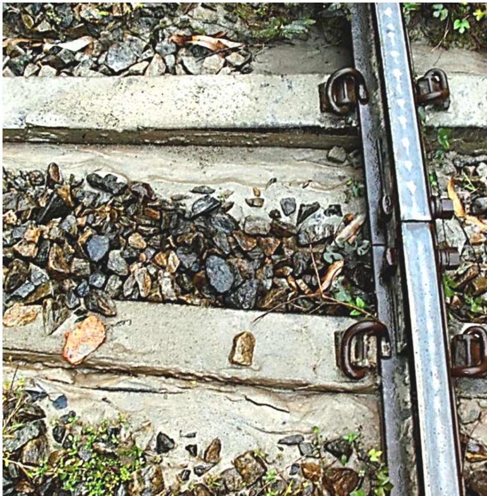
Fig. 12: Typical “Mud-Pump” of “dancing Sleepers” on SLR Track; Pict. by F. Wingle
