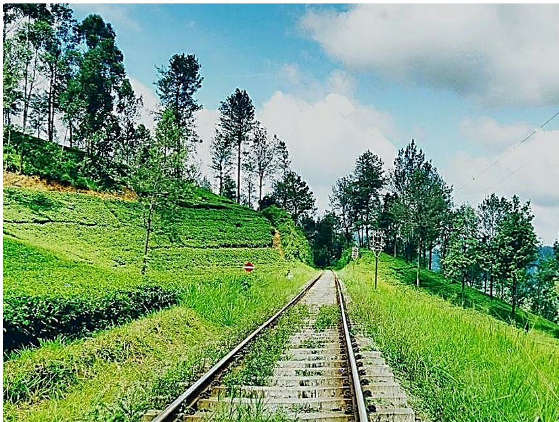
Fig. 26: The only Broad Gauge Main-Line Track around the Globe with Concrete Sleepers laid on a poor bearing Formation with nearly no Ballast Cushion; SLR Upcountry/Uva Line; Pict. by Ceylon Railway Forum
