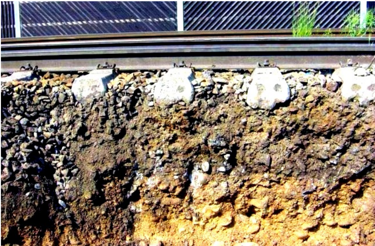
Fig. 9b: Ballast and Formation-Material are mixing due to insufficient Ballasting and missing Formation Protective Layer, Pict. by Plasser&Theurer
