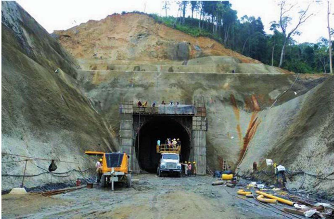
Tunnel under Construction on the Aizwal, Mizoram, Rail Project, Section Bhairabi to Sairang
