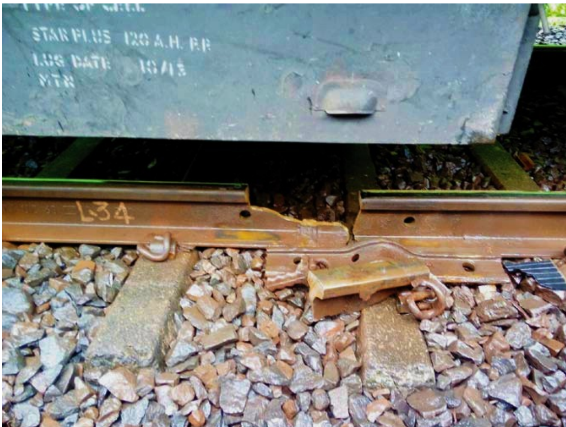
Typical in-Service Failure of a low Quality AT-Weld bandaged with Joggle Fishplates; Central Railway, Asangaon, 20 th September 2015
