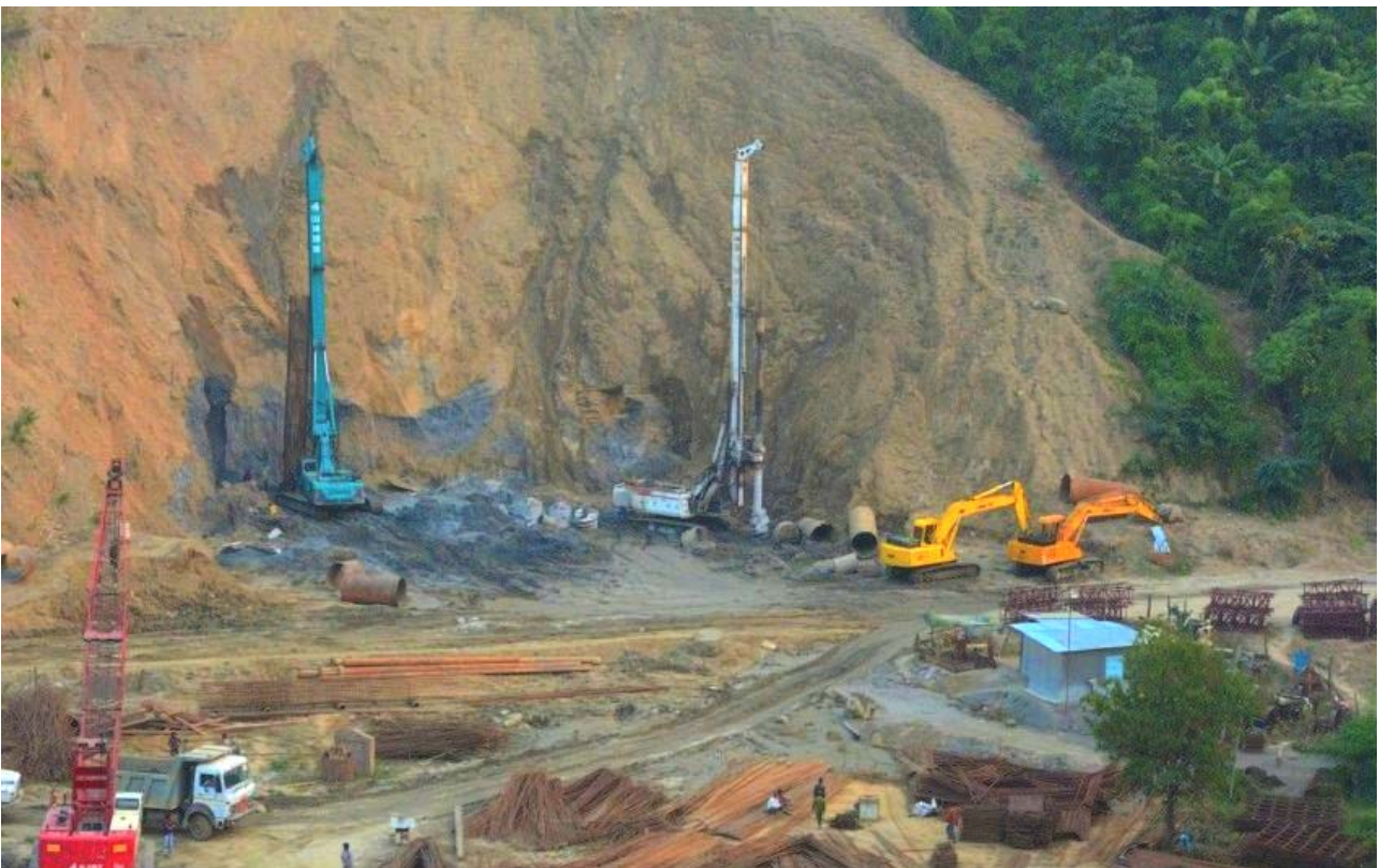
Building a new Railway Line from Jiribam, Assam, to Imphal, the Capital of Manipur
