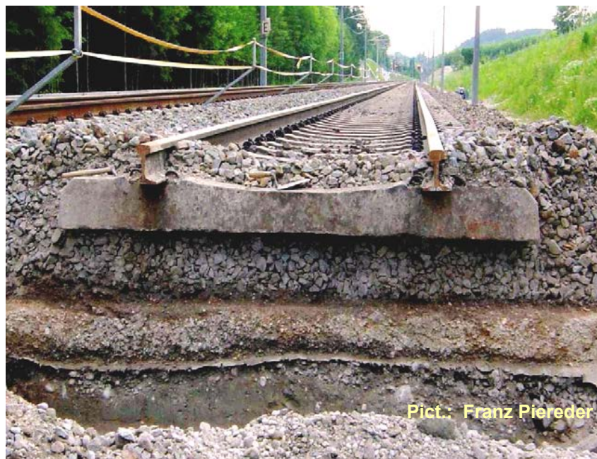
Cross-Section of a deformed Rail-Track with Strata/Sub-Grade, Subsoil, Formation protective Geo-Textile, Sub-Ballast Blanket, Ballast, Sleeper, Rail-Fastening System, Rail
