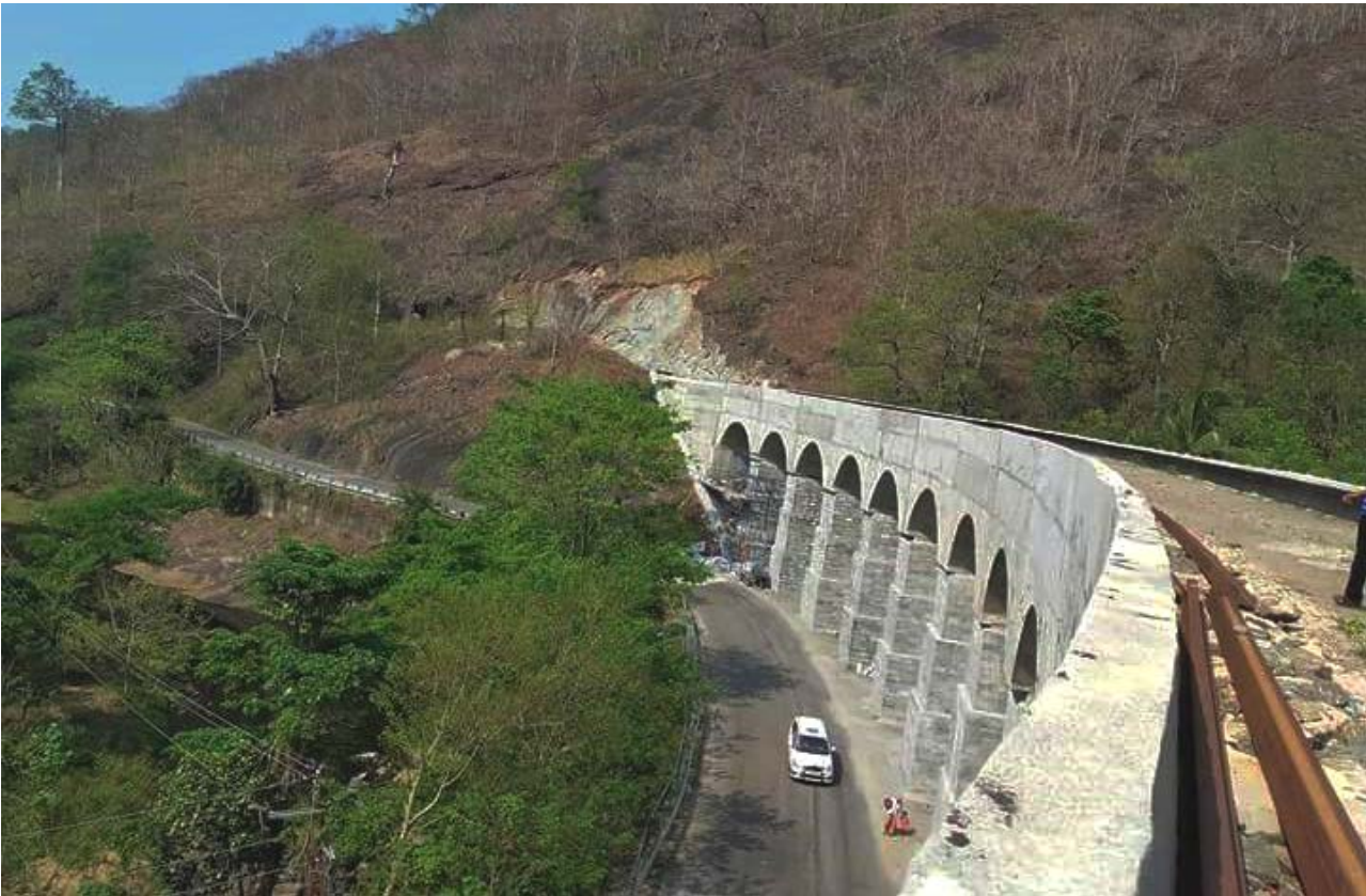
Upgrading the Kannara 13-Arch Bridge on the Kollam-Sengottai Branch-Line from Meter- to Broad-Gauge Conversion
