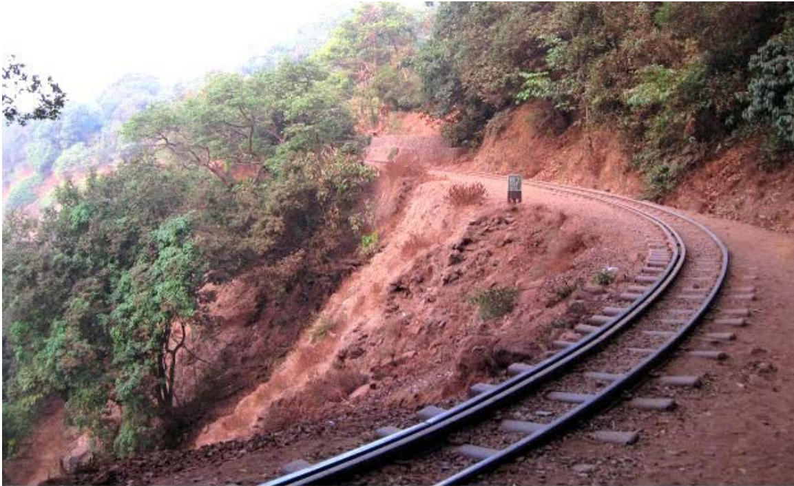
Formation flowing down the precipice between Aman Lodge and Matheran near Wayside Inn; kinking Curve Rail-Joint
