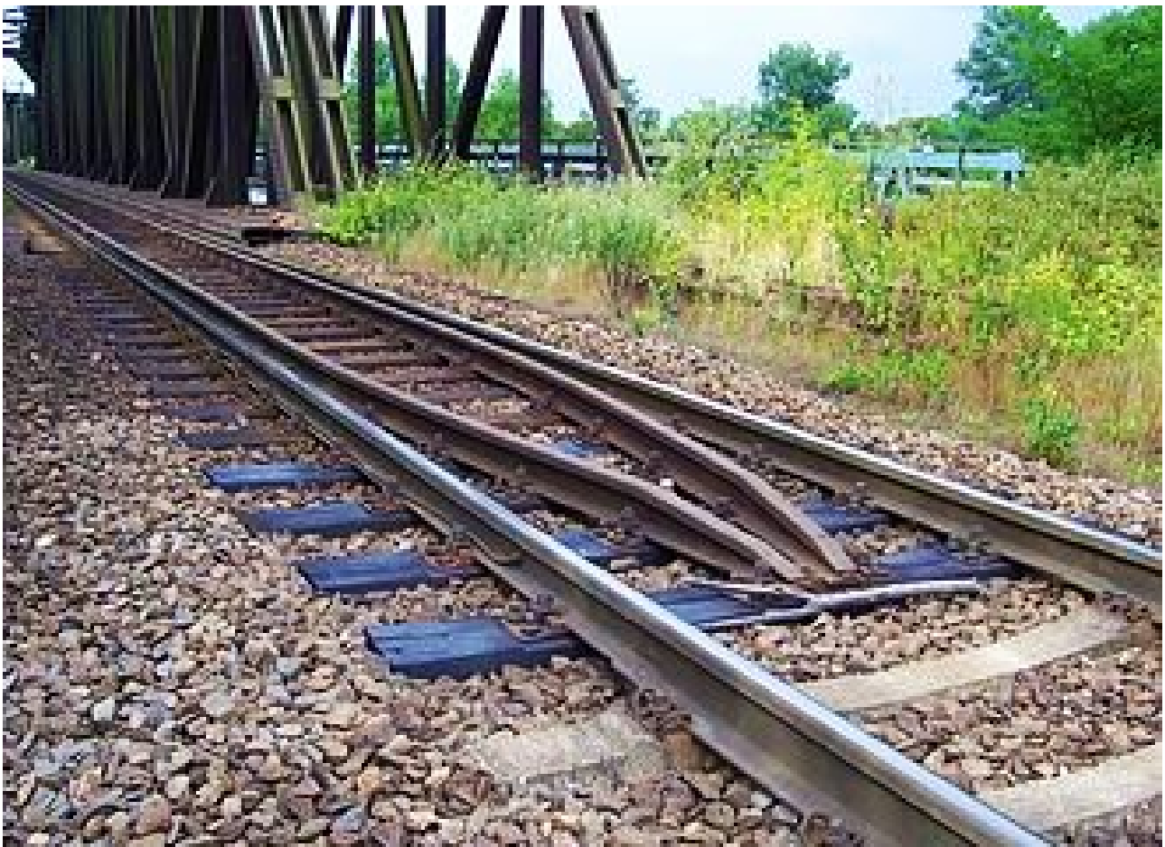
Derailment-Protection at Bridge by Guard-Rails
