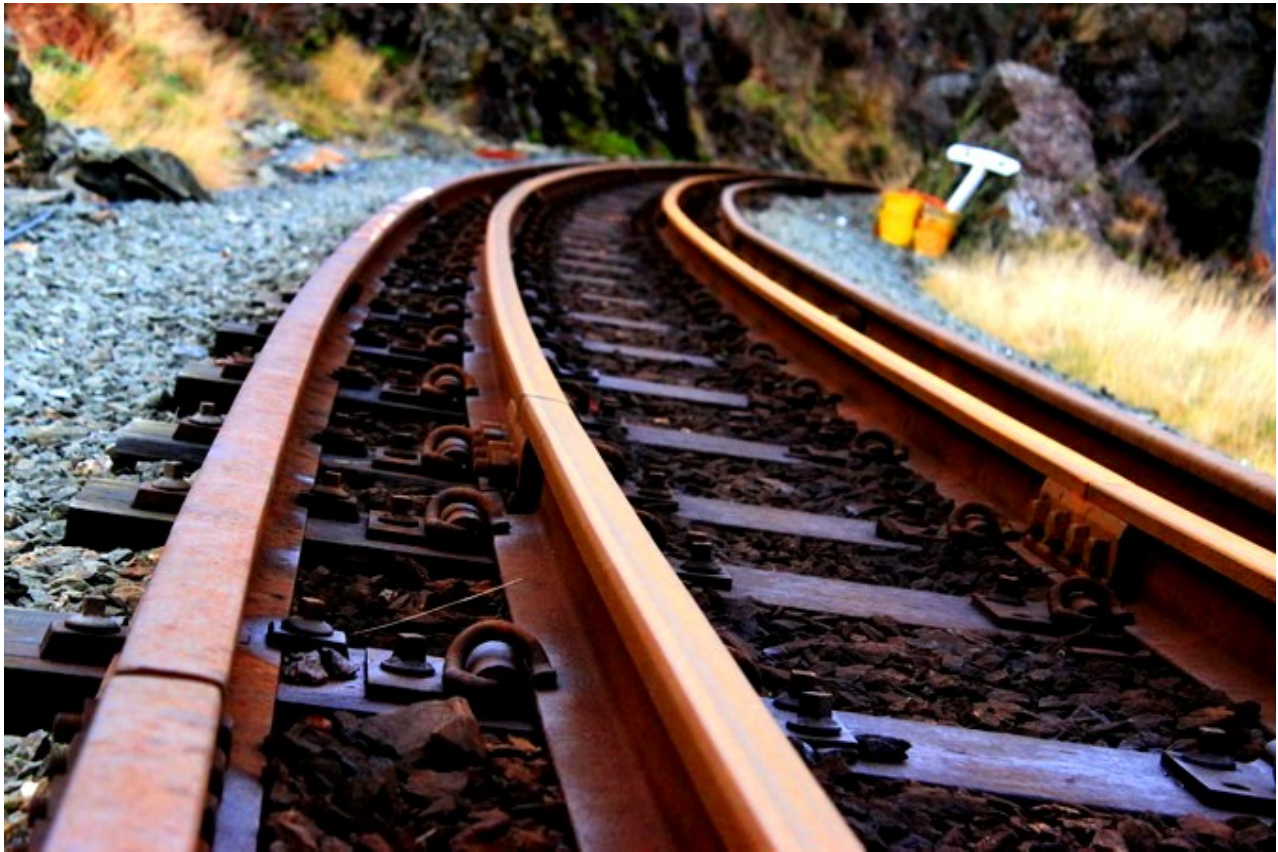
Protection at Precipices by outside Guard-Rails on 2 ft. NG scenic Festiniog Railway, Wales, England
