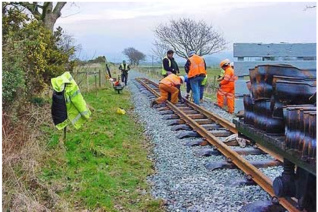
Laying 2 ft. NG Rail Track on Trough Steel-Sleepers on a well ballasted Formation; Welsh Highland Scenic Railway, Wales, England
